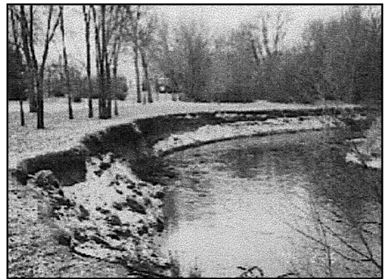
After a Heavy Rainstorm
